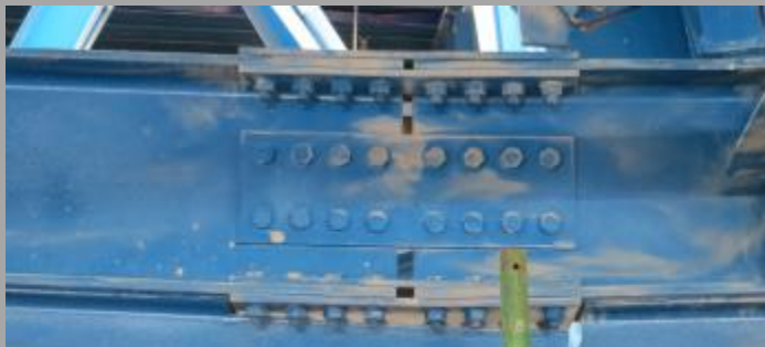
Main beam bend at connection
