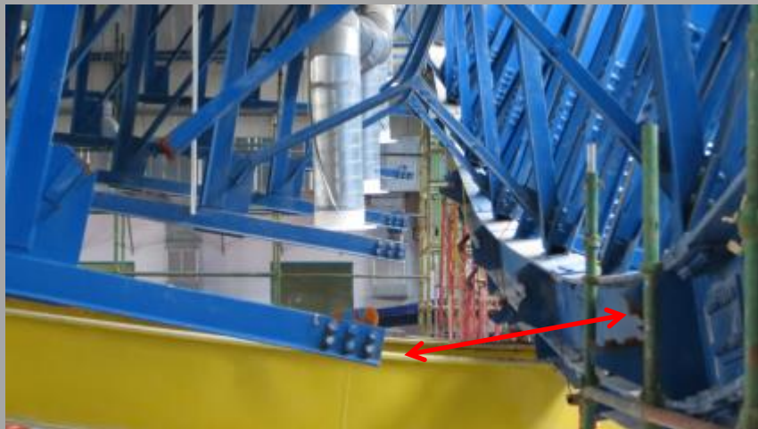
All Connection to secondary trusses broken at east side
