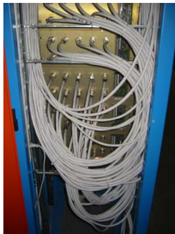
Powering Interlock Controller (PIC)
